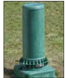
Installed 28" (749 mm) GLC with Grounding Spacer
