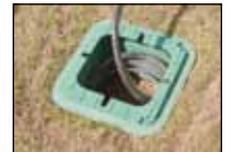
Slack Cable Storage in Small Base
