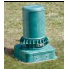
Installed 17" (453 mm) GLC with Grounding Spacer
