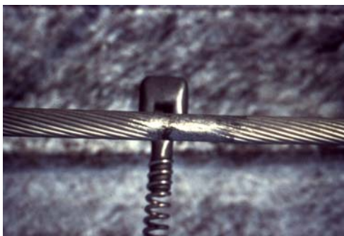
Figure 4 – Abrasion Damage at Spacer
