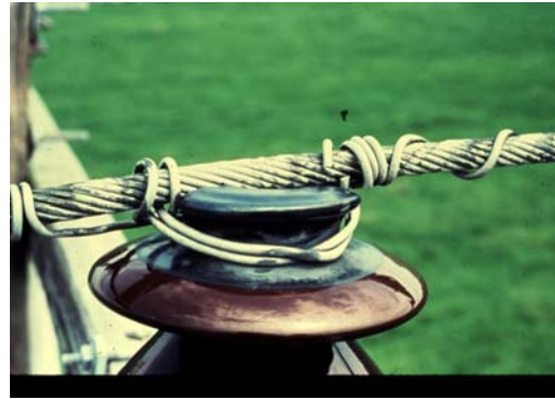
Figure 5 – Abrasion Damage at Loose Hand Tie
