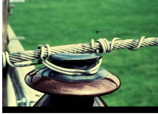
Figure 5 – Abrasion Damage at Loose Hand Tie
